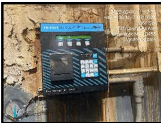
Photo 25. Low Voltage Control Panel
