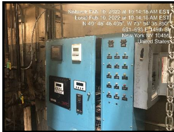
Photo 18. Boiler Control Panel
