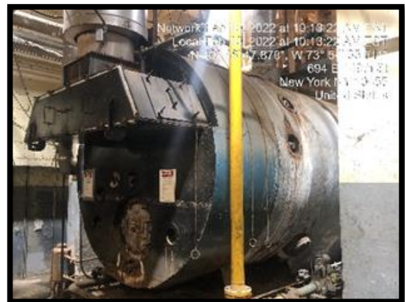
Photo 17. Current Boiler and Burner Assembly
