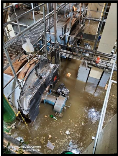
Photo 3. Moore House Building 1 Flooded Basement
