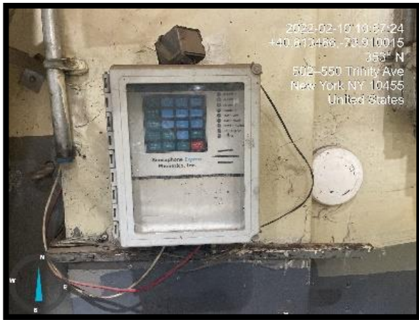
Photo 27. Low Voltage Control Panel
