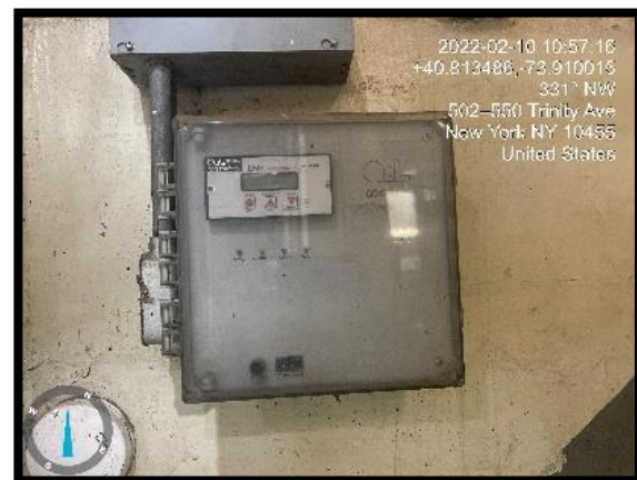
Photo 26. Low Voltage Control Panel
