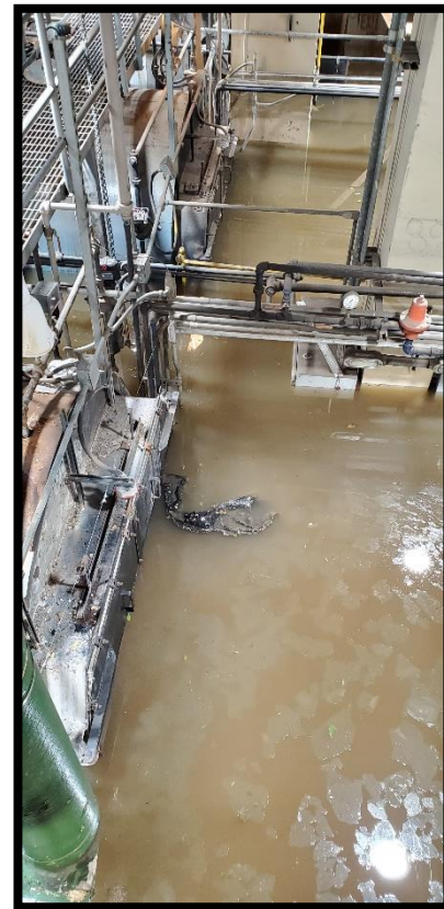
Photo 6. Moore House Building 1 Flooded Basement
