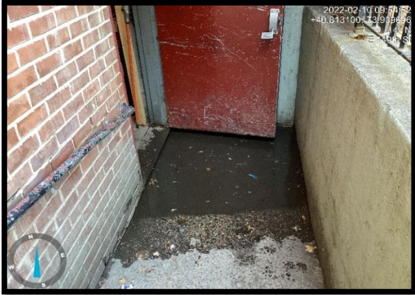
Photo 10. Boiler Room Door clogged drain During Field Visit
