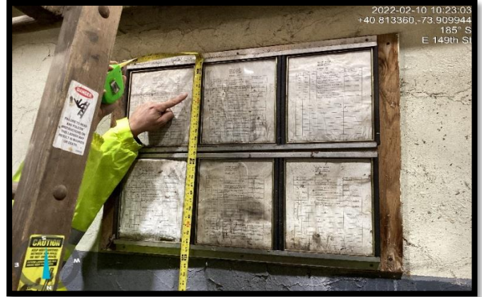
Photo 11. High Water Mark inside the Boiler Room during Field Visit
