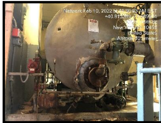
Photo 22. Domestic Water Storage Tank
