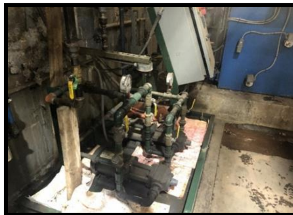
Photo 19. Fuel Oil Pumping System
