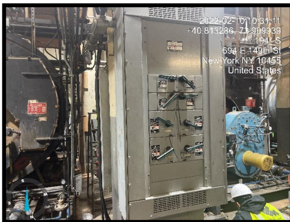
Photo 29. Power Distribution Panel Board
