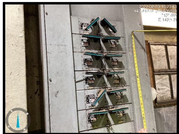
Photo 30. Miscellaneous pumps Vacuum pumps panel (208 V 3 Phase — 400 Amps max) and High Water Mark
