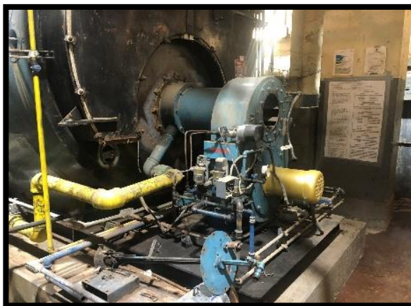
Photo 16. Current Boiler and Burner Assembly
