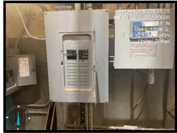
Photo 32. General Electrical Panel
