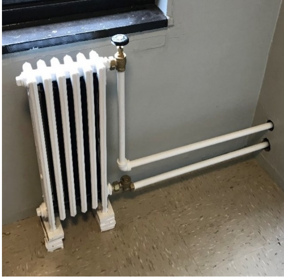
Existing conditions: exposed radiator pipe and poor mounting
