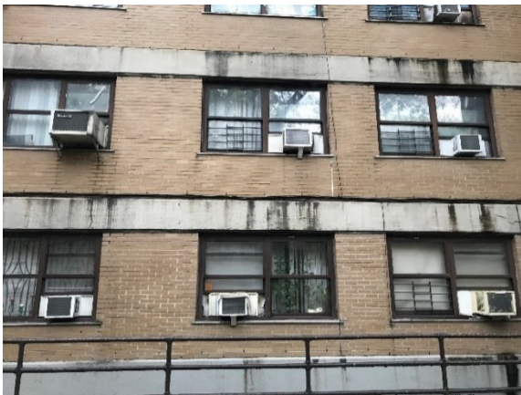
Existing conditions – facade staining
