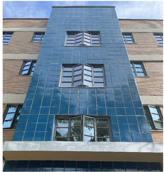
Williamsburg: Improved façade that conceals wiring and cables.
