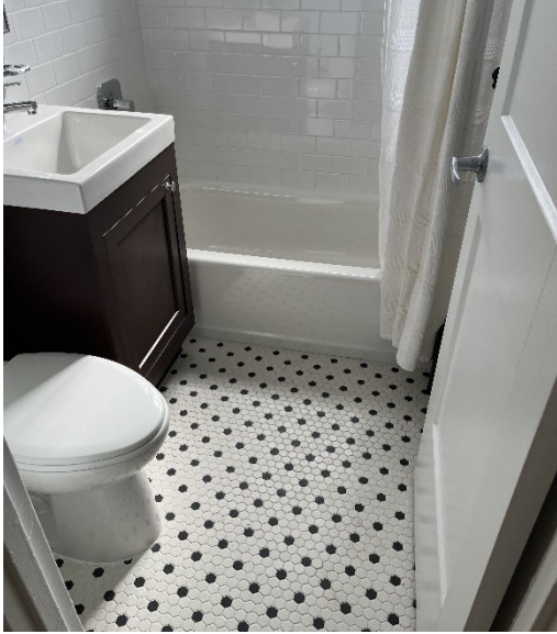
Williamsburg: Vanity, tub, full height tiling
