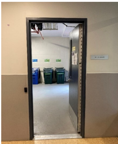
Project: Baychester and Murphy Houses; Dedicated recycling room
