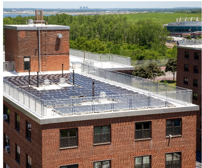
Ocean Bay Bayside: Solar panels
