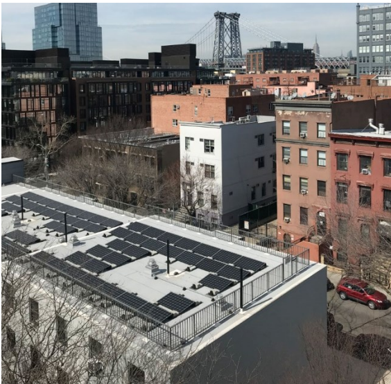
PACT Brooklyn Bundle: Solar panels and cool roof
