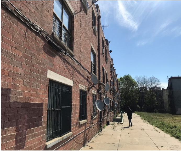
Existing conditions – exterior wires and satellite dishes
