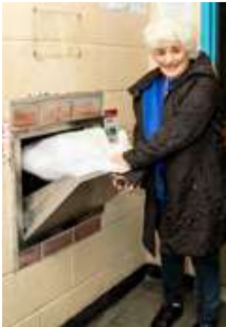
Top: Old hopper doors are too small for kitchen garbage bags.
