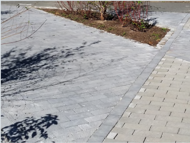
Stone pavers and planting area installed for Edenwald Houses Green Infrastructure Program
