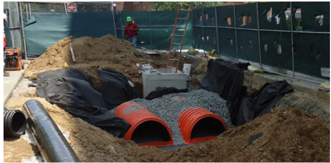
Subsurface infiltration systems are installed underneath parking lots or other large paved surfaces. They include a bed of broken stone and a storage system, such as storm chambers or perforated pipes.
