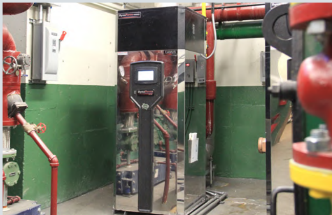
Condensing gas boilers are much more energy efficient than their steam and hydronic counterparts. Installation at Hope Gardens.
