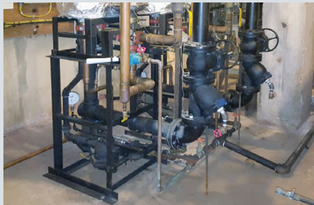
Instantaneous hot water heater at Carver Houses
