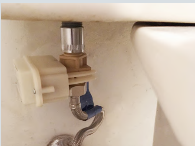
Wireless water leak detection meter installed on the ultra-high efficiency toilets to monitor and collect water usage data. Photo: H2O Degree
