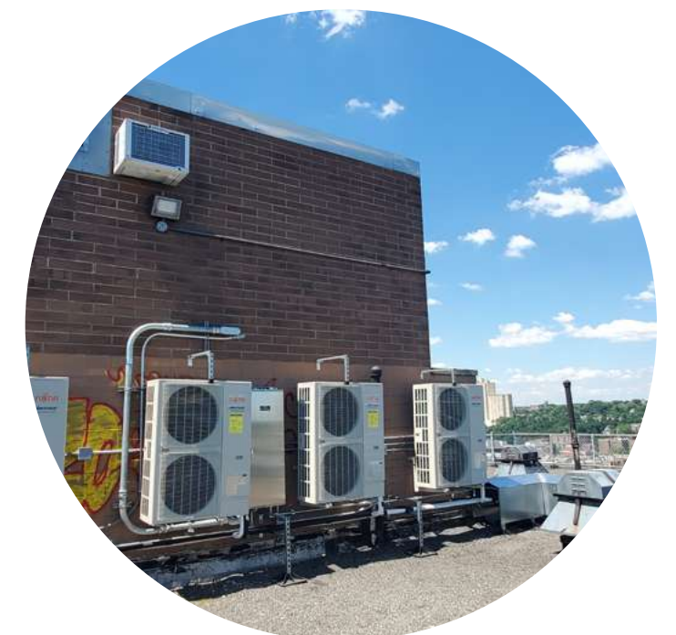
Outdoor units of heat pump system in Fort Independence.
