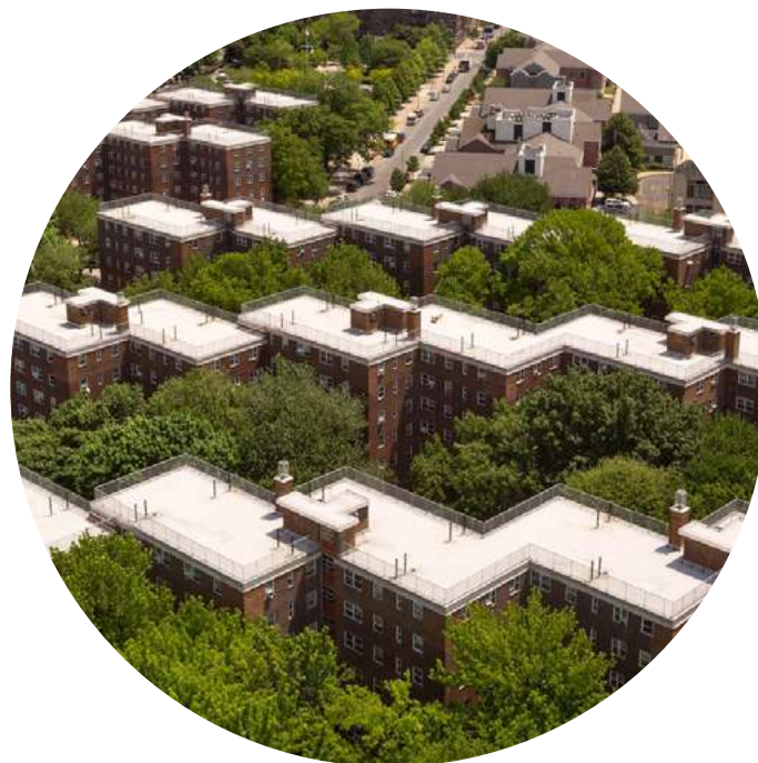
Kingsborough Houses underwent exterior renovations which included façade repairs, asbestos abatement, brick replacement, parapet replacement and reroofing.
