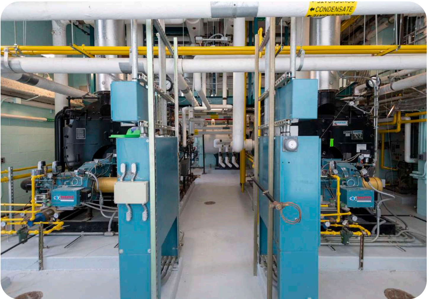
Boiler room in Coney Island 1B
