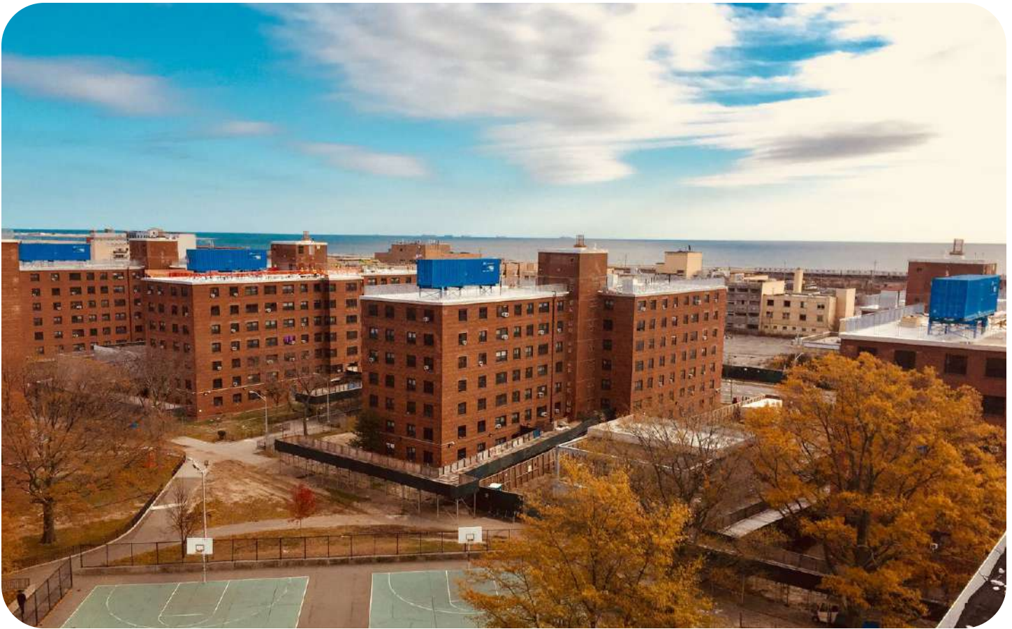
Hydronic Boilers on the roof at Ocean Bay Bayside
