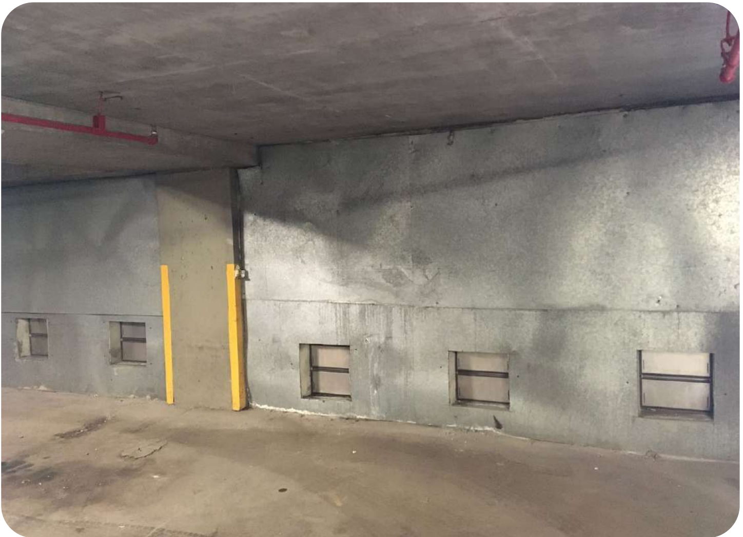
Two Bridges: the parking area has vents in order to wet floodproof
