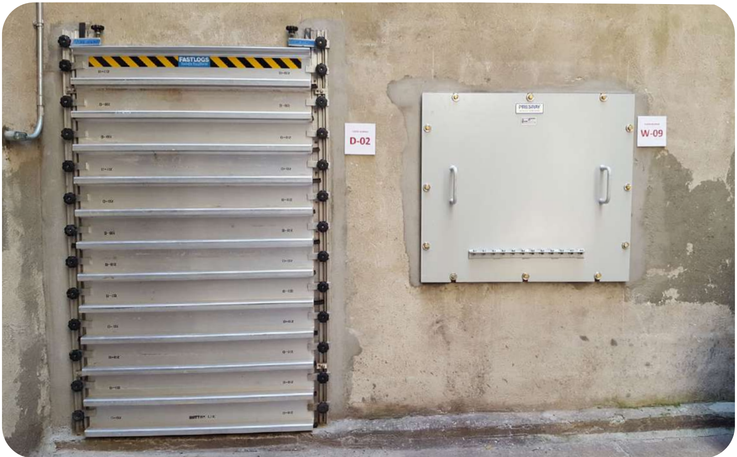
At Lower East Side V, site constraints required critical infrastructure be protected in existing below grade spaces
