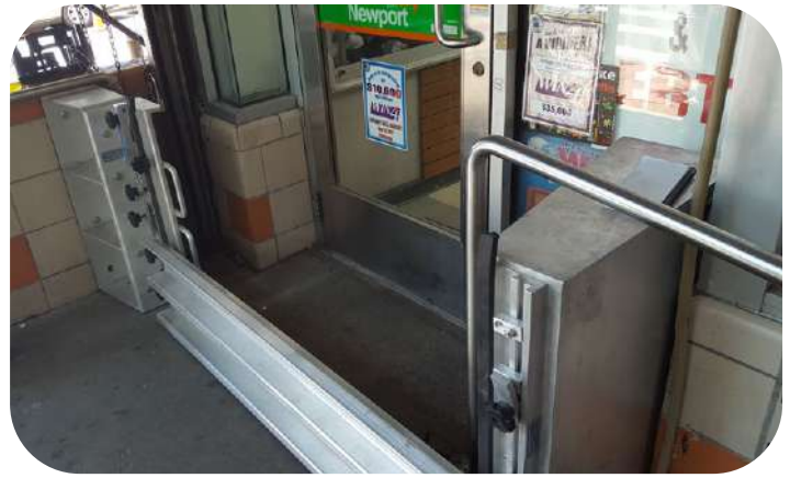
Lower East Side V: Deployable flood panels in front of a store
