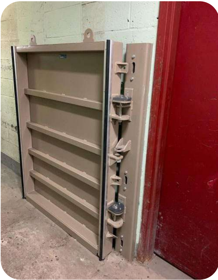
Two Bridges: Flood door in a hallway in the basement to delineate a protected zone
