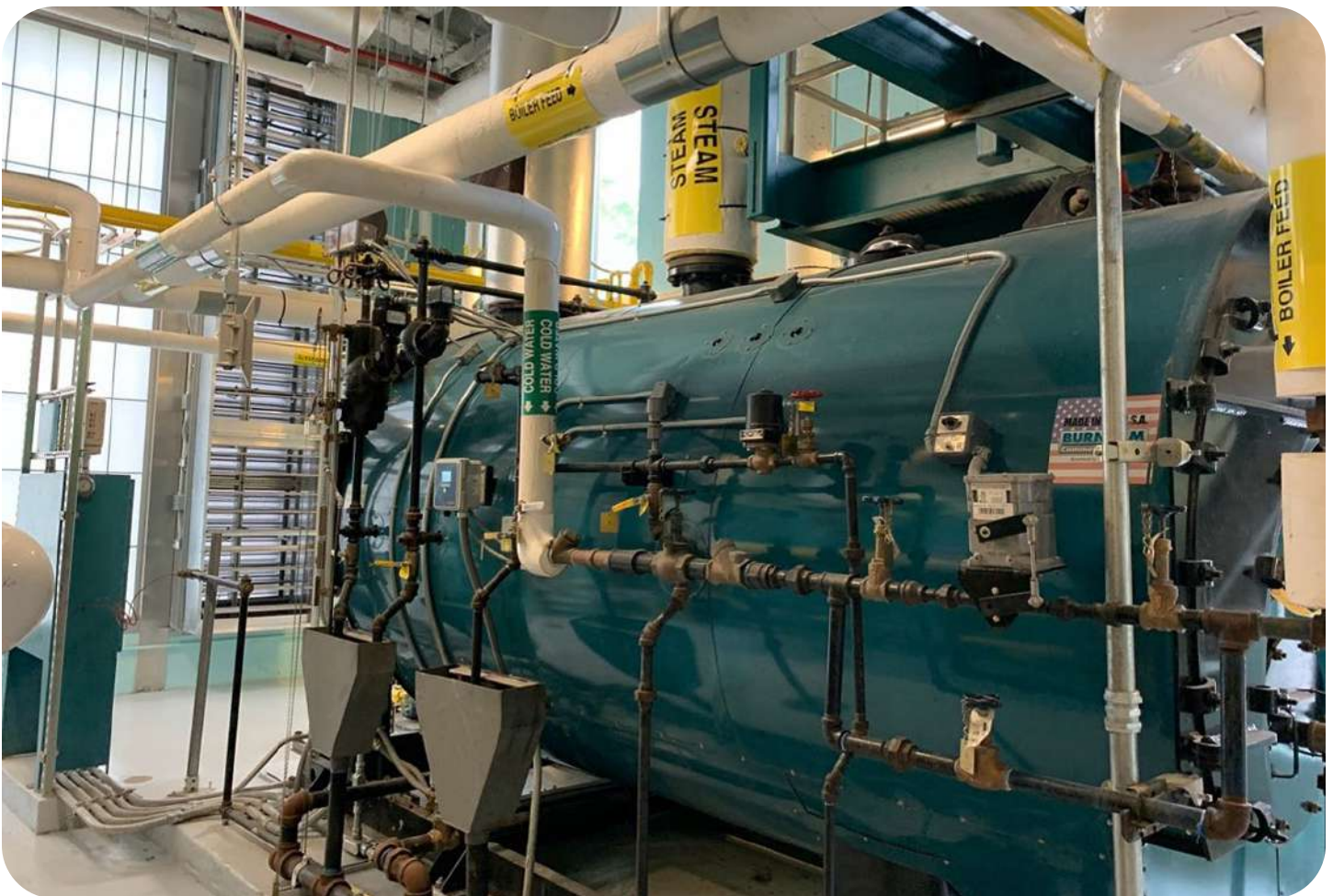
Boiler room in Coney Island 1B
