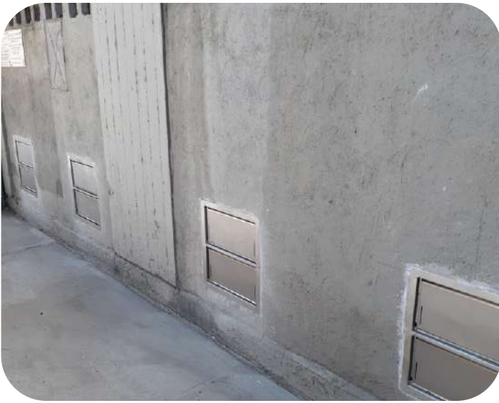
Two Bridges: wet floodproofing vents seen from the outside of the building
