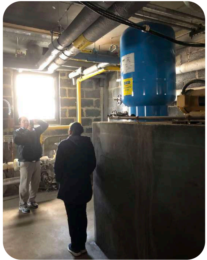
Raised equipment at Ocean Bay Oceanside
