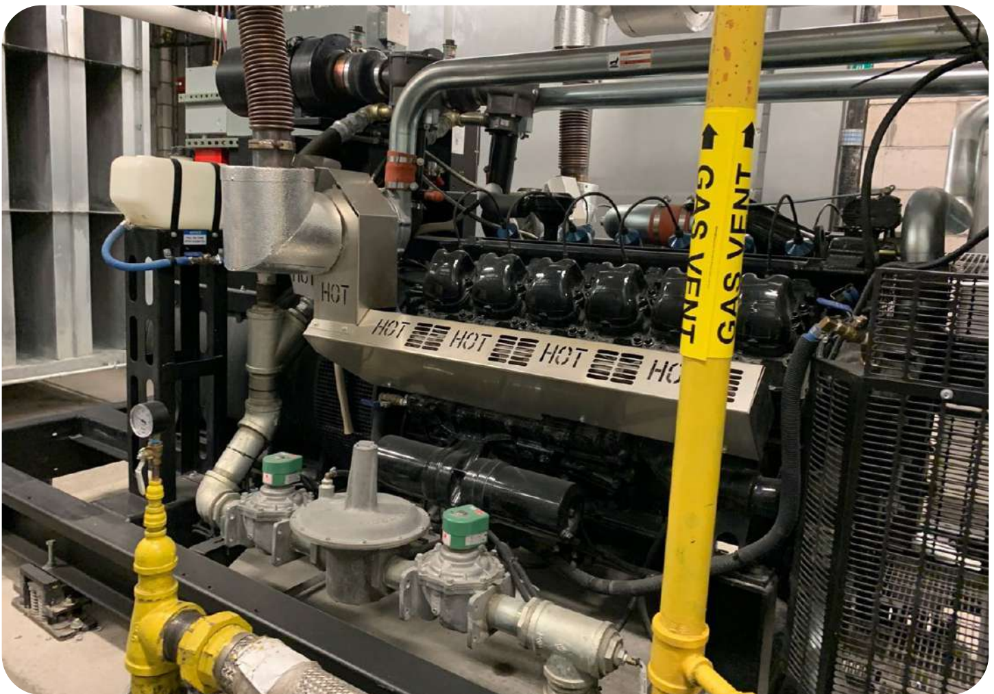
Newly installed backup generator at Coney Island 1B
